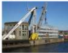
Figure 75. Emergency Bullhead Crane System at Chickasaw Lock - South District, United States Army Corps of Engineers - The system is used for setting bullheads in front of the lock structure under flow conditions. The system is also used for maintenance dewatering.
