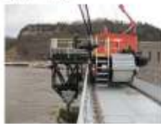
Figure 76. Lock and Dam 9 Mississippi River - Salt and Sand District United States Army Corps of Engineers - The undercarriage of the crane incorporates the bullhead lifting equipment. The lifting beam on crane is utilized for setting maintenance bullheads in front of the dam gates - These systems are utilized for balanced maintenance on the bullhead.
